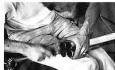
Jardine's system required some work with ballpeen hammer and file before the pipes would go into the collector.
